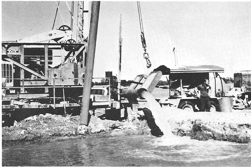
Hydrogeological assessment, not divining, led to the construction of this bore. It is tapping water-bearing gravels at a depth of about 124 metres in the Murrumbidgee Valley and is shown here being pump tested at 150 litres per second.
